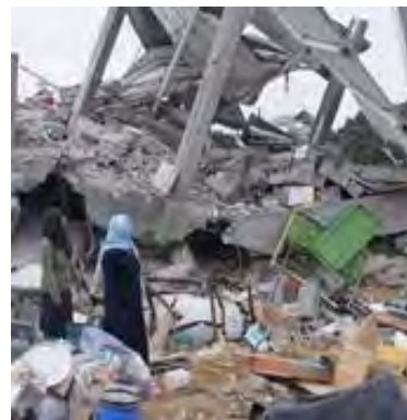
Figure 2: Home Demolition - Izbat Abd Rabo, Gaza
